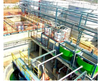
ZLD Based Effluent Treatment Plant with Reverse Osmosis (RO) and Multi Effect Evaporator (MEE) Technology
