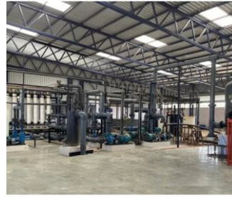
Effluent Treatment Plant and Water Treatment Plant
