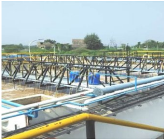
Effluent Treatment Plant and Sewage Treatment plant on Extended Aeration Technology
